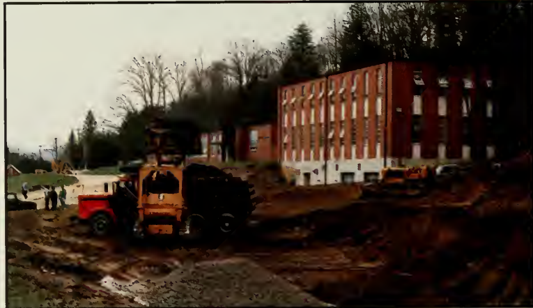
Because of the growing Industrial Education and Technology Department, a new wing will be added to Kerr Scott Hall.
