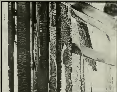
Charred timbers and an empty brick shell are all that remain of Ivy Hall.
