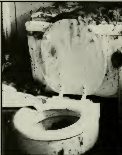
An electrical fire caused by faulty wiring in a vent fan began in this bathroom.
