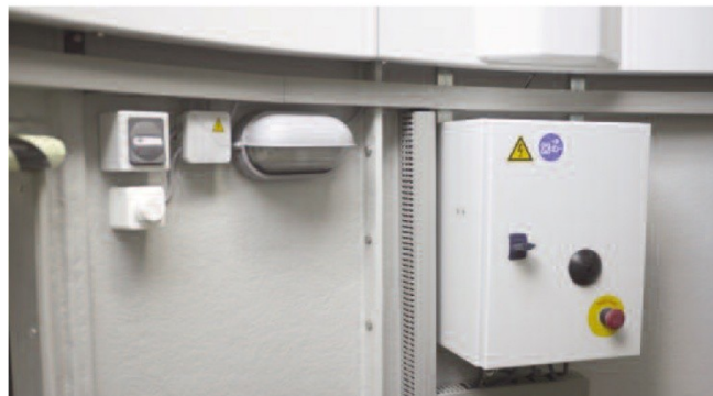
A tidy impression: electrical installations in the dome
