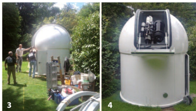
(3) Completion of base and dome; (4) Finishing of the assembly work with built-in instruments
