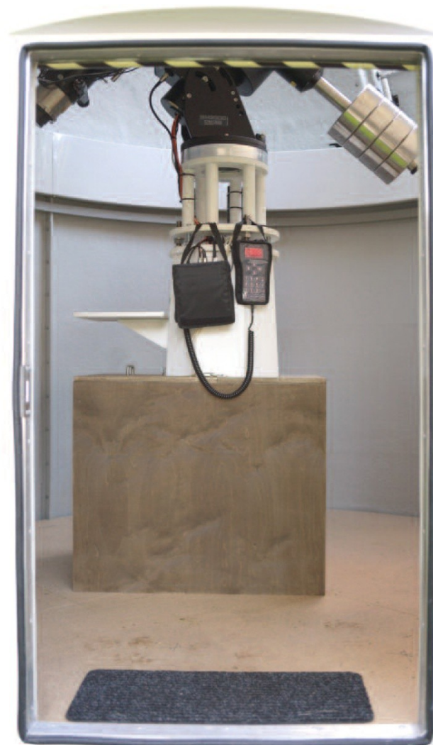
View through the door from outside: the wooden base around the heavy column takes power supply units and the extensive cabling of the instruments, eyepieces and cameras.
