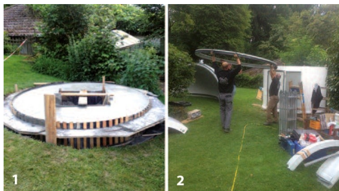
Installation in June/July 2014: (1) double foundation for observatory and column; (2) installation of dome ring
