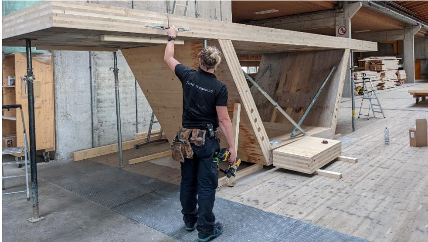
Figure 18: Manufacturing box-girder modules at the factory. Picture: Flück AG, Wangen b. Dübendorf
