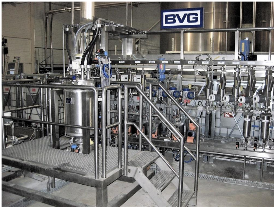
Continuous Operating BVG Coating Kitchen “Super-C-Shear” at Hamburger Containerboard, Spremberg PM1
