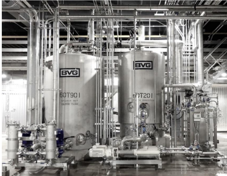
Continuous Operating Enzyme Starch Processing System BVG-Super-ECC at Pratt Wapakoneta, OH USA
