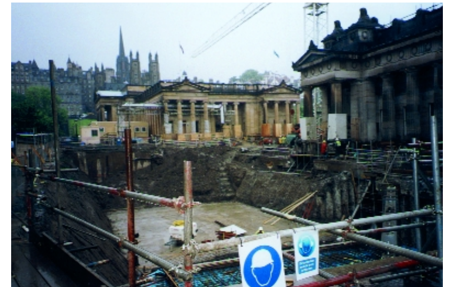
The Playfair Project in the making. This extensive refurbishing and underground linking of the National Gallery of Scotland (left) and the Royal Scottish Academy (right) will create more exhibition space and museum facilities.
