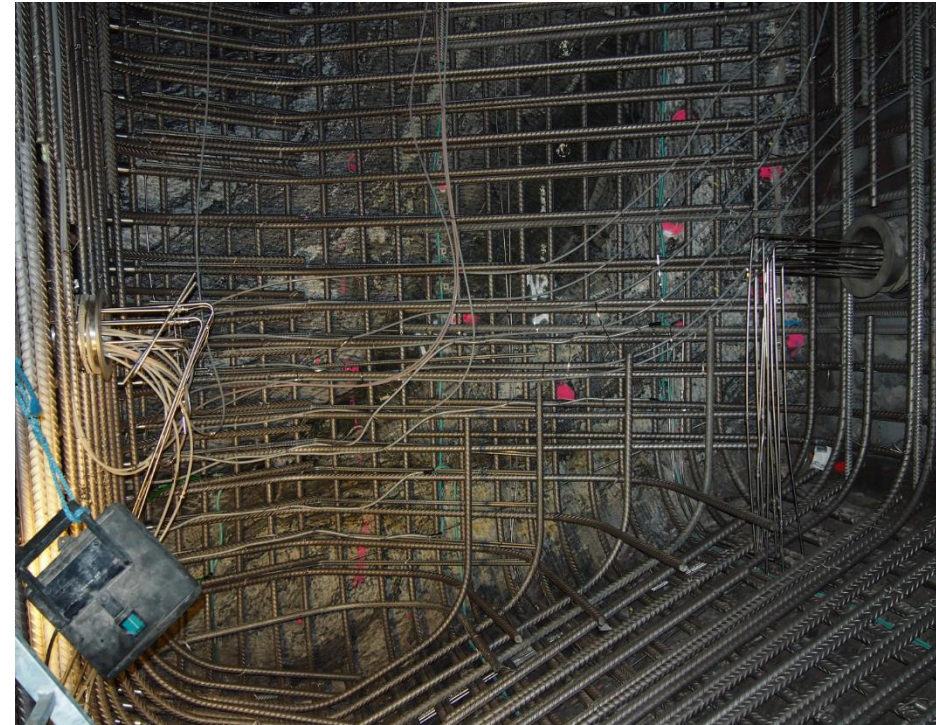
PVDF and stainless steel tubes, directing the pressure sensor cables to the cable flanges towards the filter layer (right side) and plug section 2 (left side)
