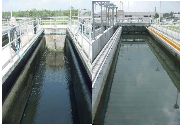
Figures 1 and 2. Denitrifying filters at the East Central Regional Water Reclamation Facility, West Palm Beach, Florida
