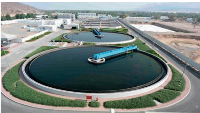
Fig. 1: Secondary Clarifier of the wastewater treatment plant of Fujairah, United Arab Emirates (UAE) (Photo: EW)
