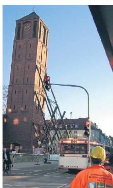
Figure 1.6: St.-Johann-Bapist Church victim of today's (none existing) Project Management [Der BauUnternehmer]
