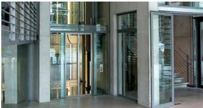
Lift fixings, guide rails
