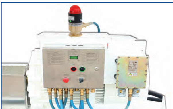
Local control unit
