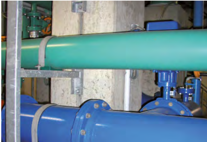
Pipe supports on vertical HZA Channels
