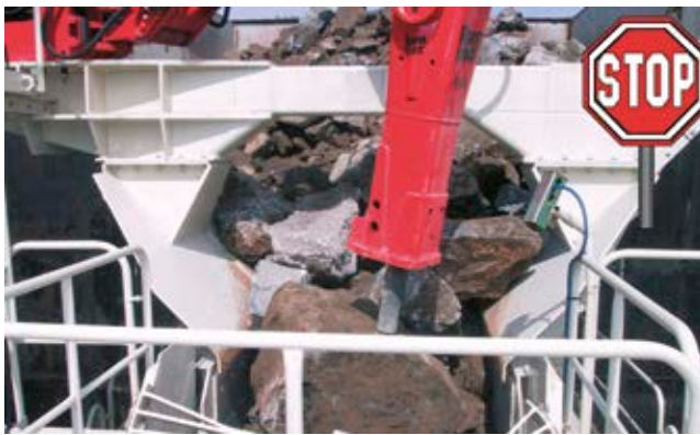
Figure 7: No oversize breaking in crushing process
