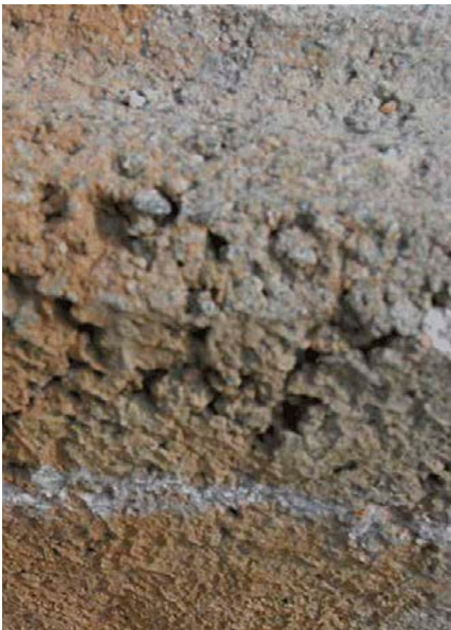
Poor concrete flow.
