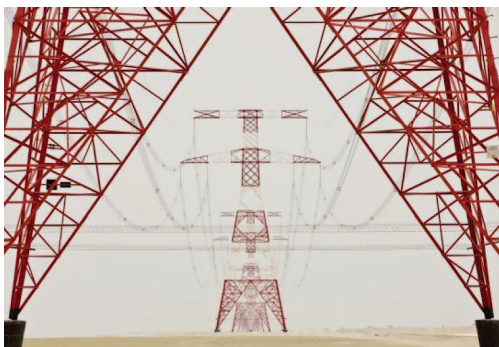
High-voltage line with spacer dampers
