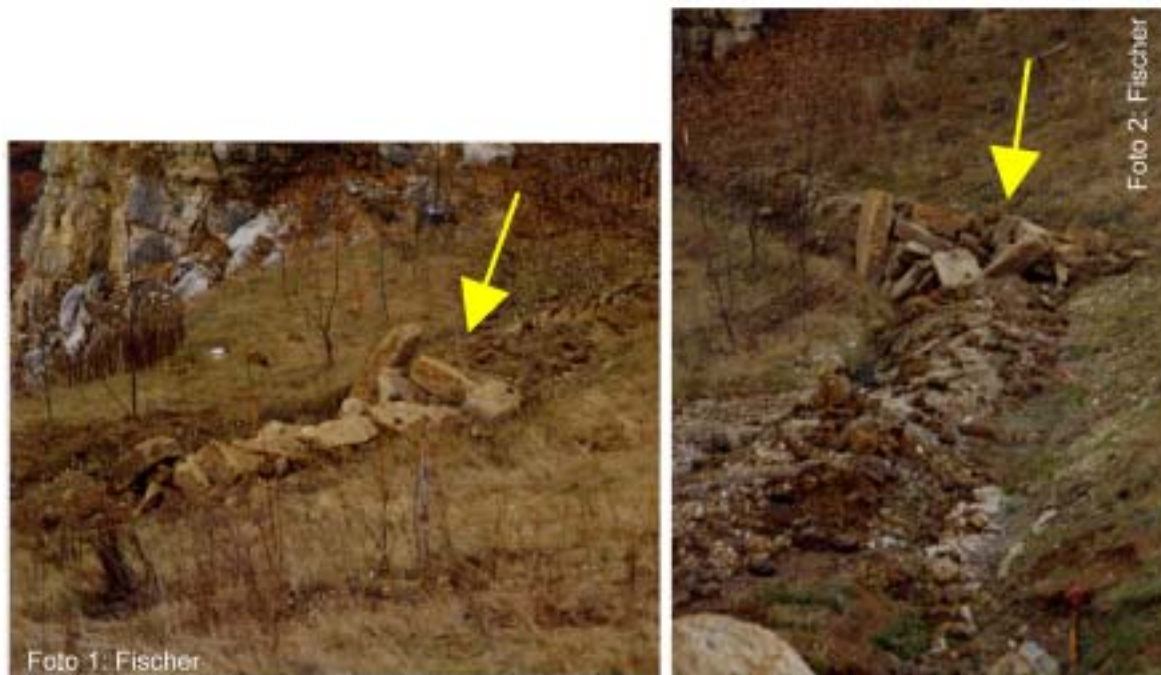
Fig. 3: Deformed natural stone wall
