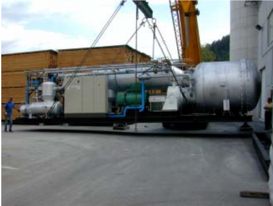
Figure 29: ORC plant in Admont (Source Bios Bioenergiesysteme)
