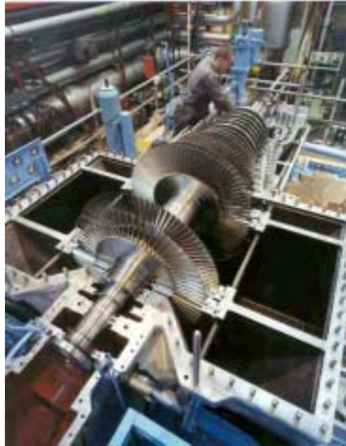
Figure 6: Rotor of a steam turbine with 8 MW el
