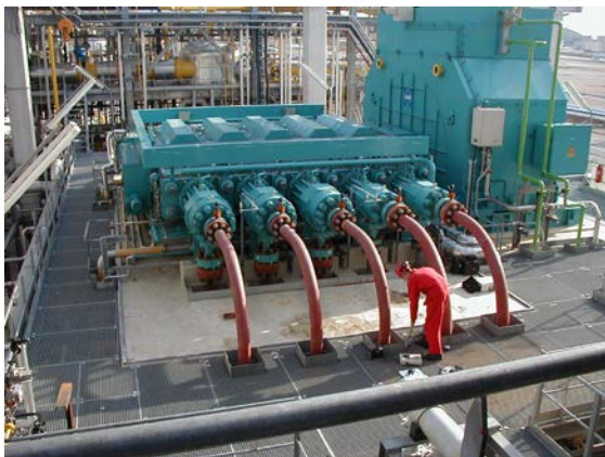
Fig. 1.1 Ethylene Hypercompressor 21 MW at Basell Aubette
