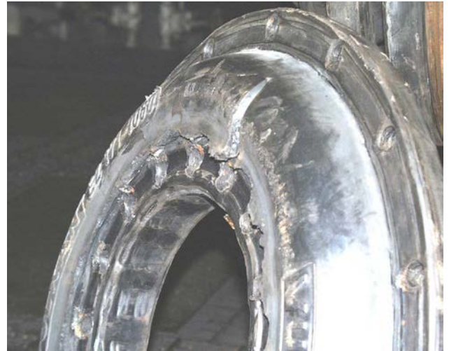
Fig: 10 – Coupling Element Damage
