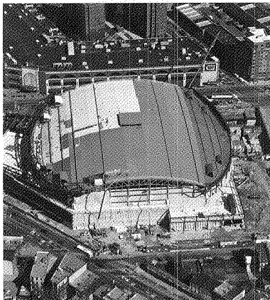
Barclays Center arena at Atlantic Yards in Brooklyn – future home of the NBA's Nets and other large-venue entertainment, events and concerts – is nearing completion and is scheduled to open in the third quarter of 2012.
