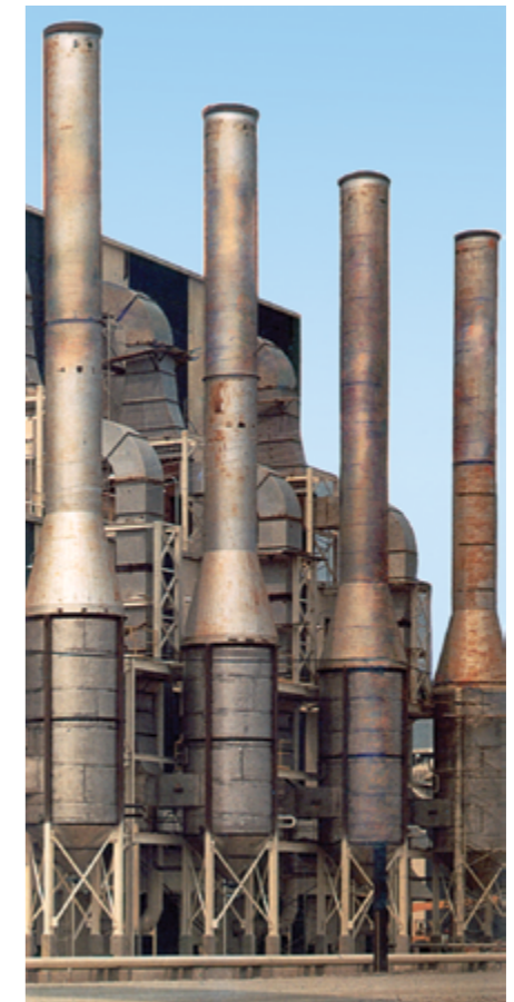
Phosphate rock calciner, USA
