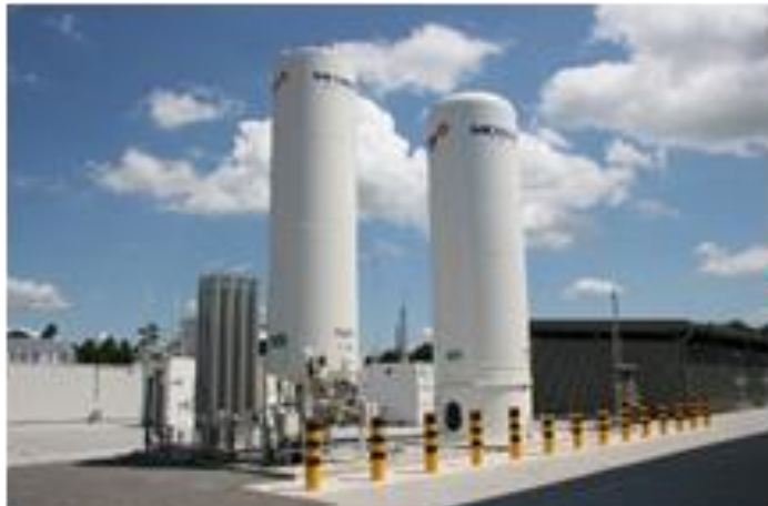
H 2 and CO 2 tanks
