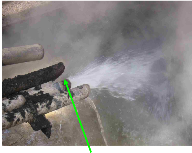
Figure 1: Hot condensate discharged into the drainage system at 98 °C
