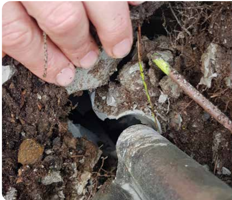
Figure 3: Damages and defects from the production of micropiles; inadequate mobility of the connection point (above); manufacturing deficiency on the top of the grout body (below)
