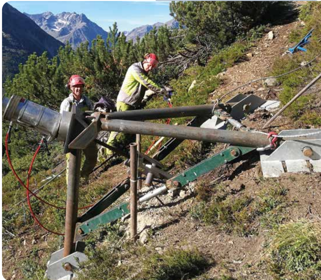
Figure 7: Inspection of micropiles at the state of the art; classic load application by press and abutment design (above, Hübner, 2019); use of specific tripod designs to the load application and inspection (below, Tartarotti, WLV)
